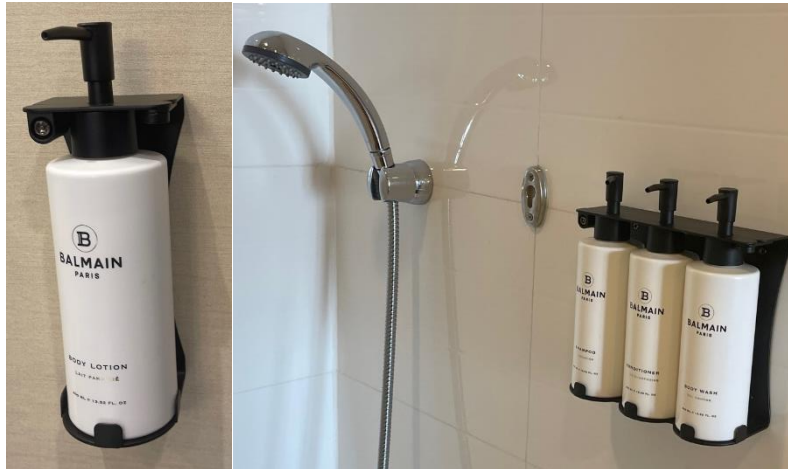
Amenity (soap, shampoo, etc.) dispensers in guest bathrooms, employee locker rooms, spa and fitness centre
